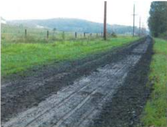
Above: Completed Phase One section of shared-use path Below: Phase One section during construction
