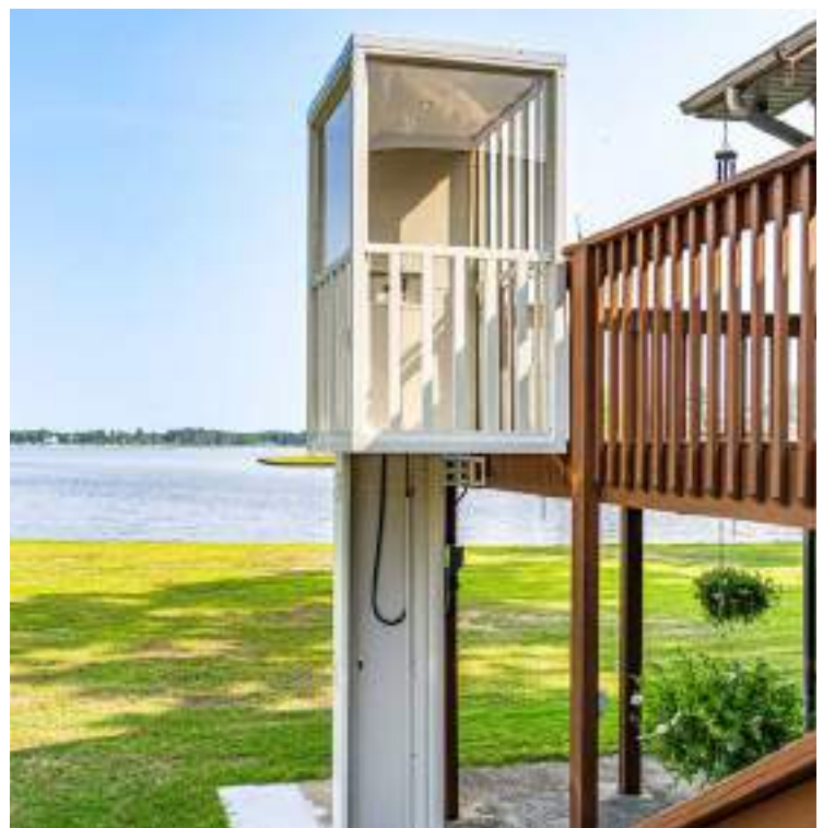
ELEVATOR FOR COMMUNITY CENTER ADA ACCESS
